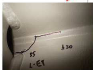
鋼床版のき裂
